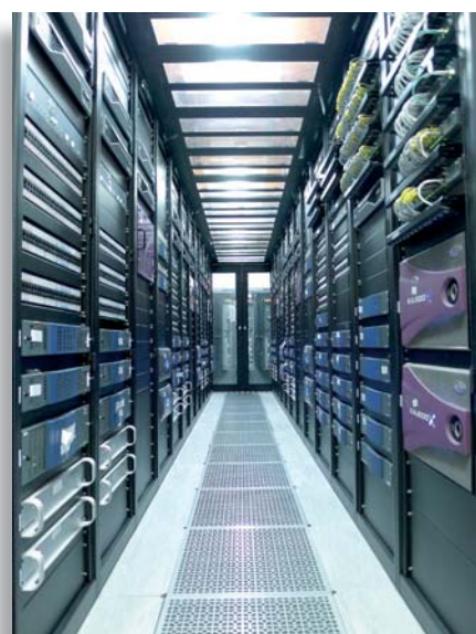
One of the five racked rooms for each of the control rooms used for CCTV's transmissions
