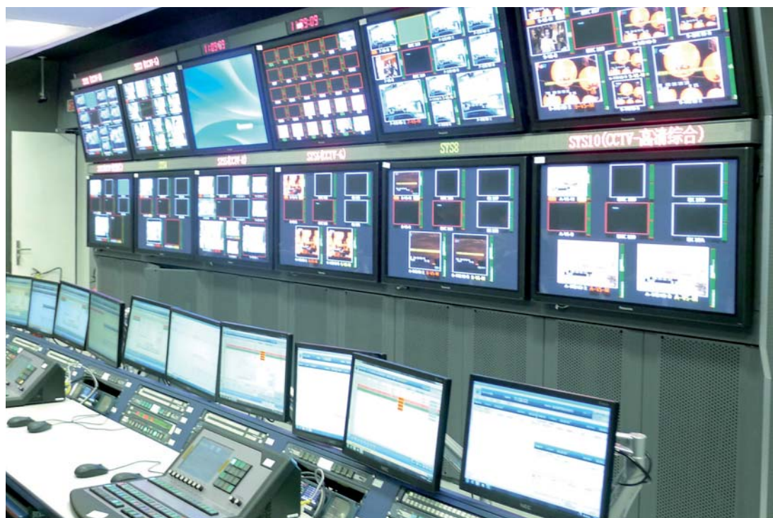
One of the five control rooms
